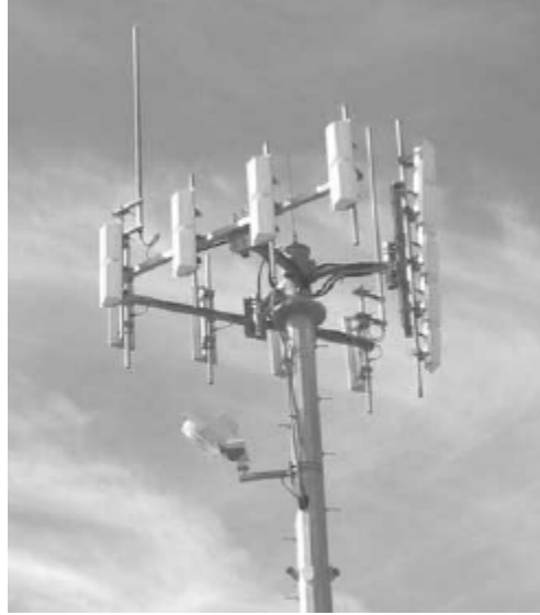
Figure 1.3: Sectorized base-station antenna
